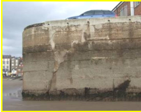
Significant cracking with exposed toe (Asset Ref. 1221D901D1301C07)
