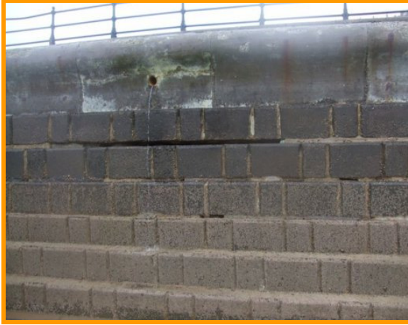
Large missing horizontal joints to wall (Asset Ref. 1221D901D1303C02)
