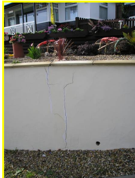
MU29/AS Cracking of a wall at Flat Cliff (Locally Active)
