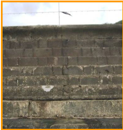
Full height vertical crack and exposed toe (Asset Ref. 1221D901D1201C03)
