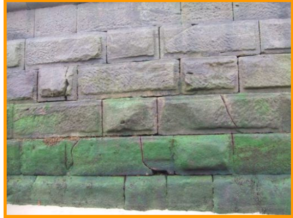
Cracking, gaps and joints and lateral movement (Asset Refs. 1221D901D0802C12)
