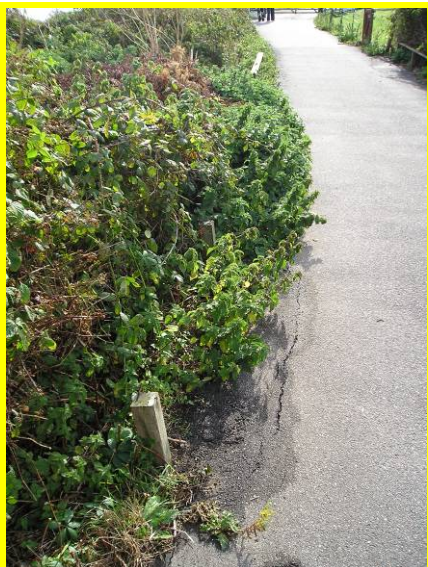
MU29/AS Minor cracks to the road at Flat Cliff (Locally Active)
