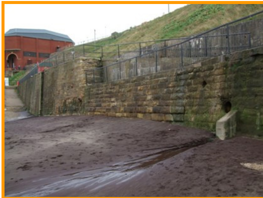
Cracking, mortar loss, damage to capping and localised repairs (Asset Ref. 1221D901D0802C07)
