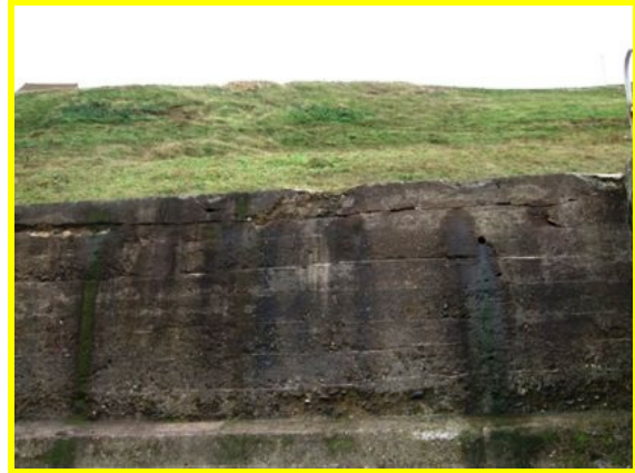
Significant damage to and cracking beneath capping (Asset Ref. 1221D901D0802C04)
