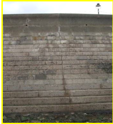
Full height vertical crack (Asset Ref. 1221D901D1201C02)
