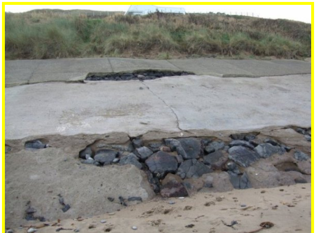
Cracks and exposed rock armour (Asset Ref. 1221D901D0702C02)
