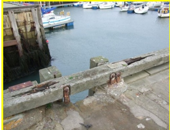
Deterioration of timber fenders throughout inner harbour (Asset Ref. 1221D901D1301C16)
