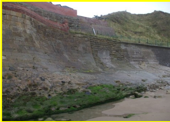
High sea defences below the pumping station, including the upper tier of red brick walls (Asset Ref. 1221D901D1402C05)
