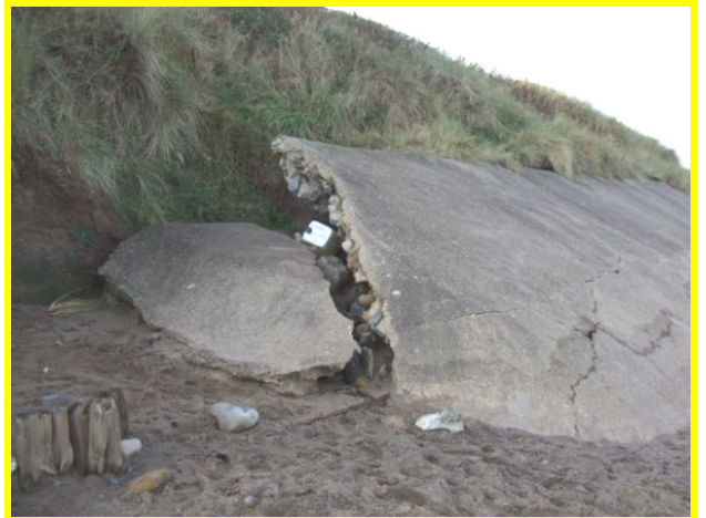
Large crack and collapse at East end of the concrete revetment (Asset Ref. 1221D901D0702C02)
