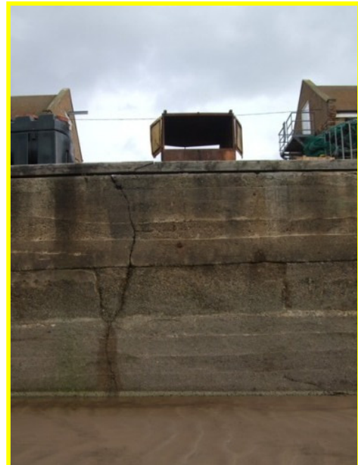
Large vertical crack extending through the wall (Asset Ref. 1221D901D1301C19)
