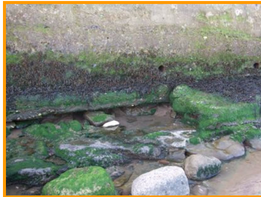
Erosion of toe near northern extent (Asset Ref. 1221D901D0802C03)
