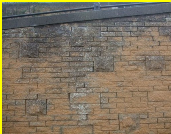
Vertical crack to second wall protecting road. (Asset Ref. 1221D901D1301C09)
