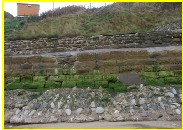
Lower section of concrete and sandstone, with joint wash out and repairs (Asset Ref. 1221D901D1402C05)
