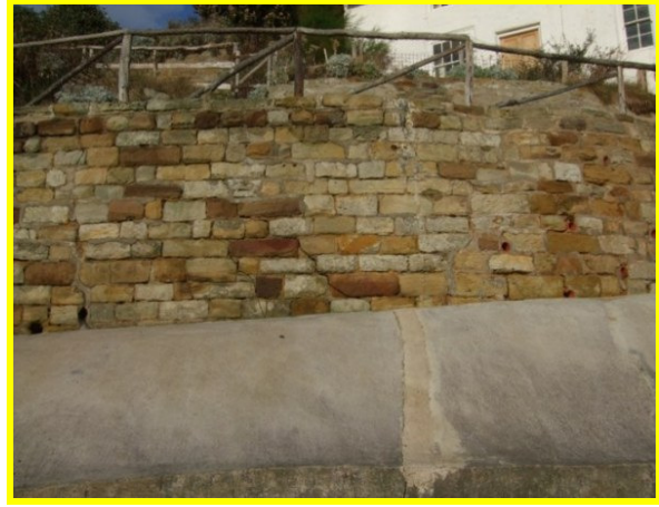
Repaired vertical crack to toe of wall and vertical cracks to second tiered wall (Asset Ref. 1221D901D0601C06)
