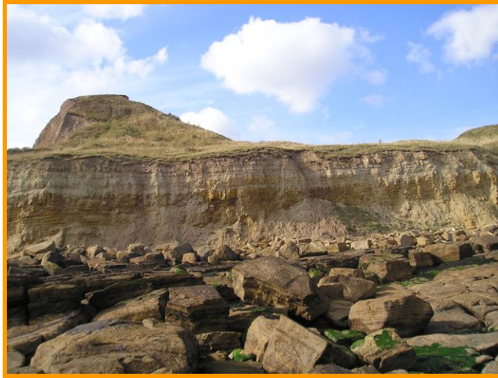
MU24/A8 Intense erosion to the east facing side of Knipe Point, and evidence of rockfall events (Partly Active)
