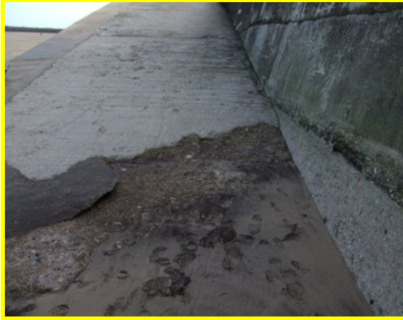
Erosion evident to slipway next to wall (Asset Ref. 1221D901D0802C13002)
