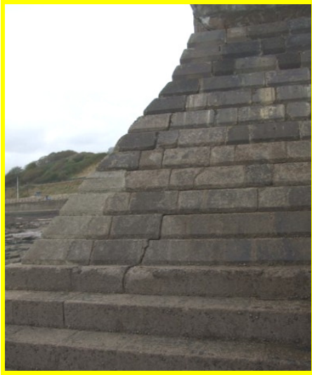
North Bay sea wall and exposed toe (Asset Ref. 1221D901D1201C02)
