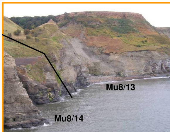
MU8/13 and MU8/14 Erosion at the toe of the units (Partly Active) (approx. extents shown)
