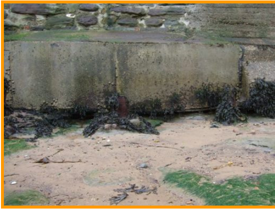
Undercutting at the toe of some parts of the harbour wall (Asset Ref. 11221D901D0402C22)
