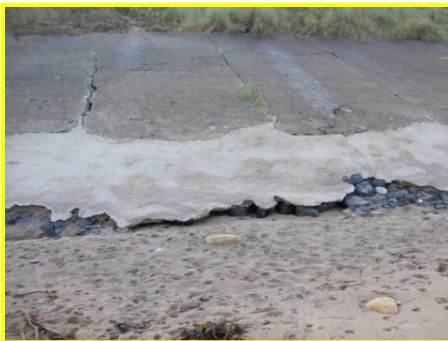
Undercutting of concrete revetment (Asset Ref. 1221D901D0702C02)
