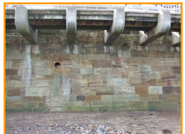
Undercutting and erosion of the concrete revetment backing Sandsend Beach (Asset Ref. 1221D901D0702C04)
