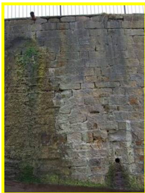
Visible joint washout and seepage (Asset Ref. 1221D901D0802C06)
