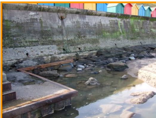
Erosion of toe and stair foundation (Asset Ref. 1221D901D0802C03)
