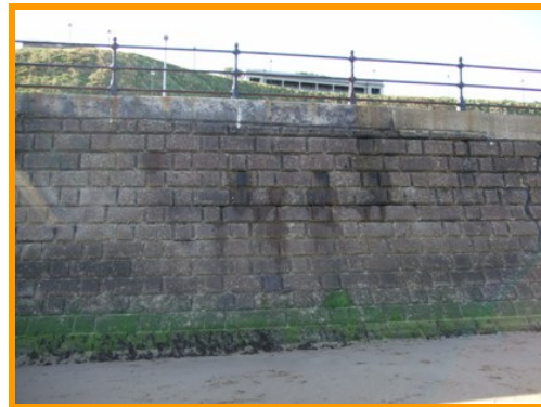
Seepage through wall and open joints (Asset Ref. 1221D901D1201C07)
