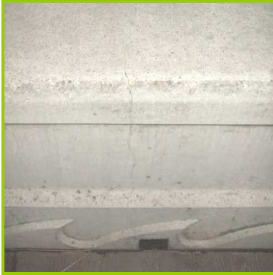
Example of crack through centre of raised wall (Asset Ref. 1221D901D1202C03)
