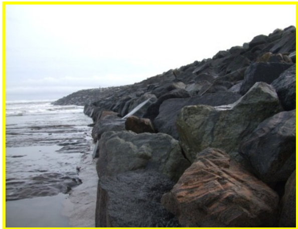
Rock armour lines the seaward side of the breakwater (Asset Ref. 1221D901D0402C01)
