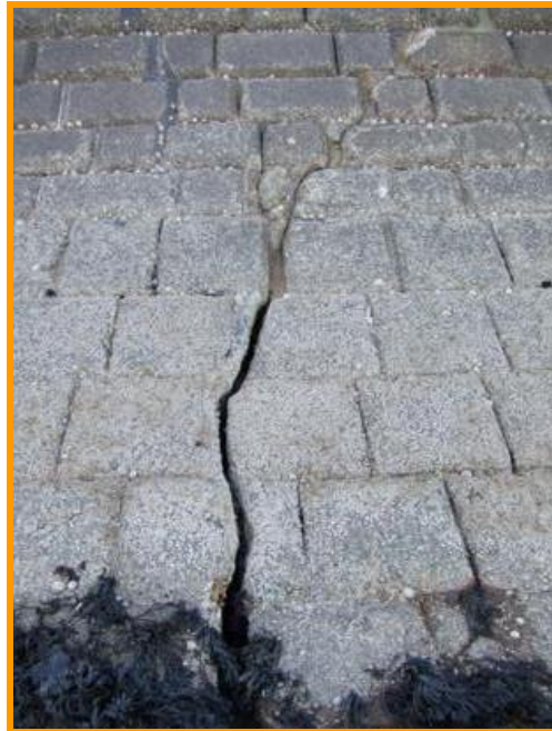
Second large crack and deep void in slipway sea wall (Asset Ref. 1221D901D1201C21)
