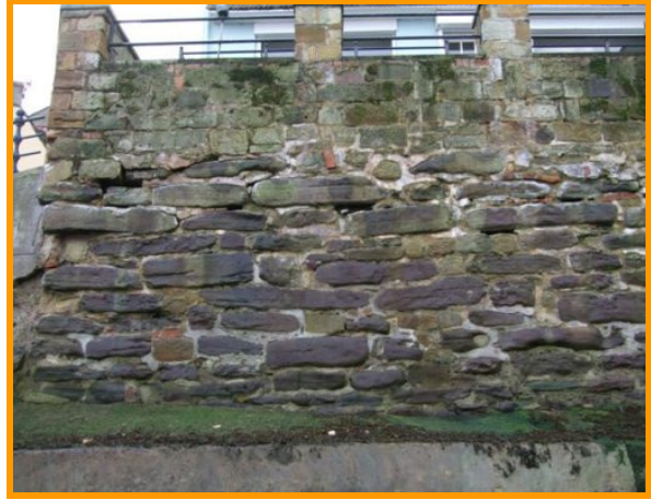
Older sections of harbour wall in need of regular maintenance (Asset Ref. 1221D901D0402C22)
