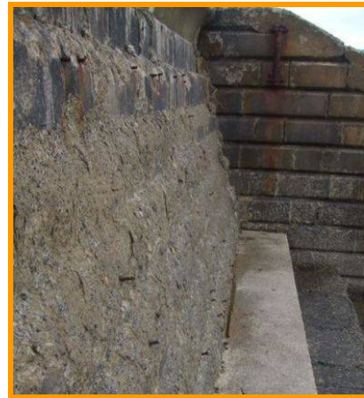
Eroded and abraded front face, exposed steel (Asset Ref. 1221D901D1201C03)
