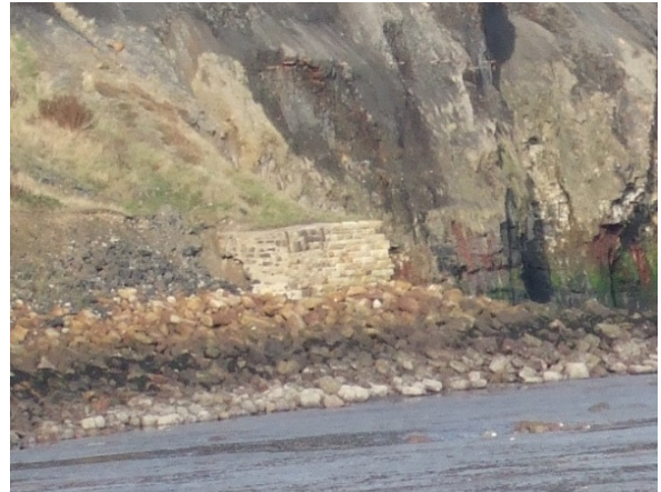
Failed masonry wall South of The Scar (Asset Ref. 1221D901D0701C01)
