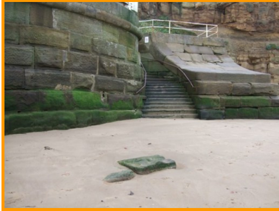
Repairs visible, also voids and gaps (Asset Refs. 1221D901D0802C12)
