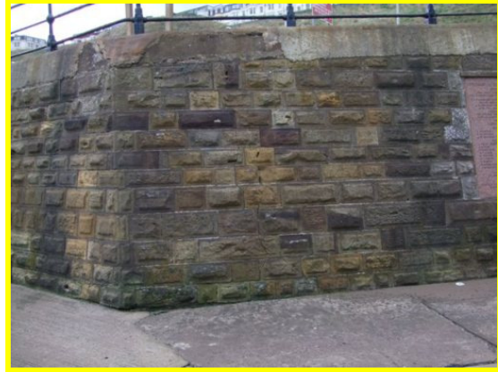
Full height cracks to left and right of corner of secondary wall beyond promenade (Asset Ref. 1221D901D1202C23)
