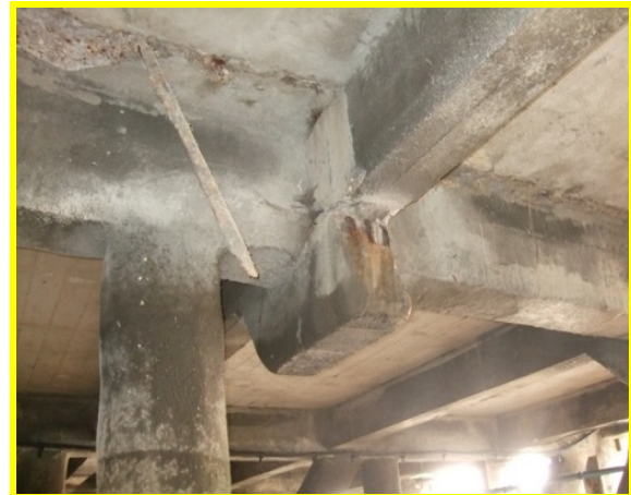
Exposed re bar and erosion to the concrete jetty supports. (Asset Ref. 1221D901D1301C06)
