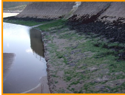
Exposed toe (Asset Ref. 1221D901D1201C21)
