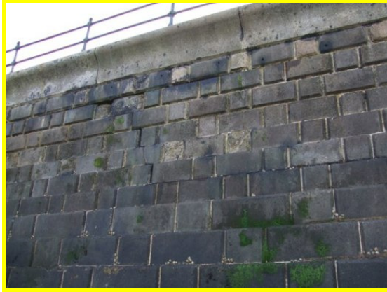
Example of cracking (Asset Ref. 1221D901D1202C23)
