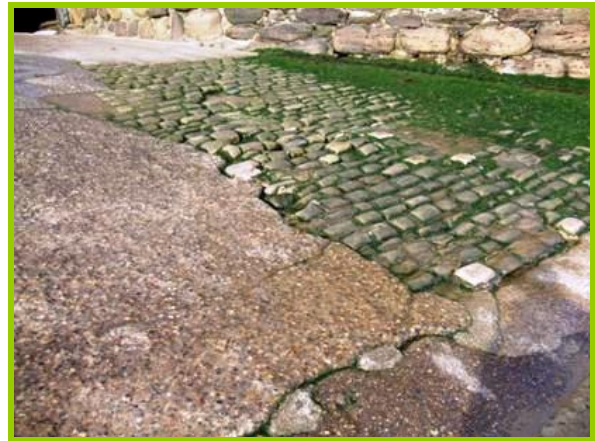
Slipway with missing cobbles and cladding (Asset Ref. 1221D901D1003C05)
