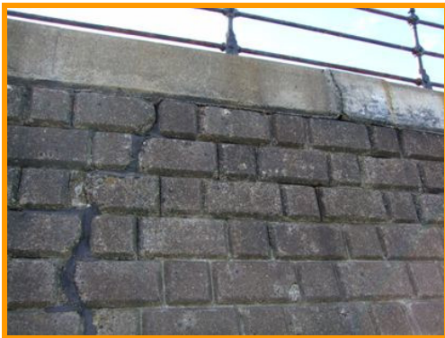
Example of repaired and re-opened crack (Asset Ref. 1221D901D1201C07)
