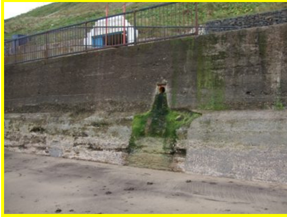
View near tunnel showing damage resulting from erosion and abrasion (Asset Ref. 1221D901D0802C04)
