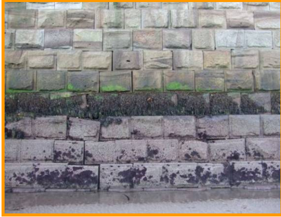
Displacement of blockwork to west side of the west harbour Pier (Asset Ref. 1221D901D0803C02)
