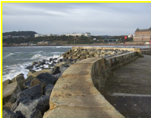
The new harbour wall with rock armour, tetrapods and raised section (Asset Ref. 1221D901D1301C01)
