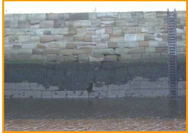
Crack and voids to east harbour pier (inspection below the water line is necessary before replacement of blocks) (Asset Ref. 1221D901D0803C03)
