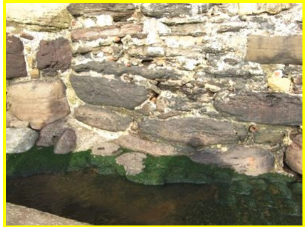
Open joints and voids visible in several places (Asset Ref. 1221D901D1003C04)
