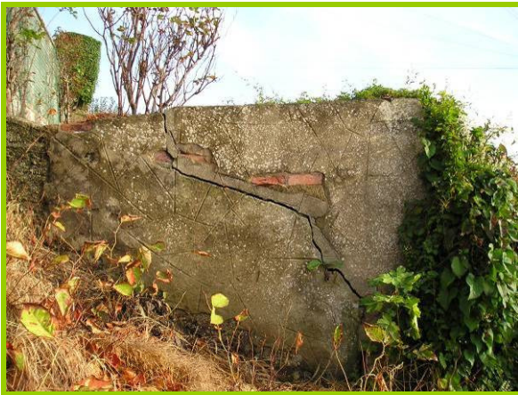
MU28/Y Cracking to wall (Inactive)
