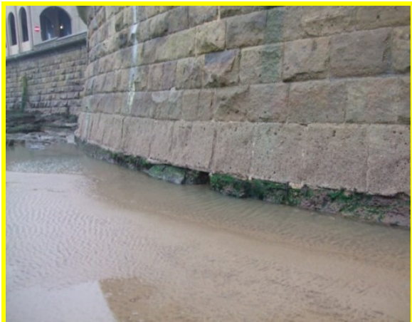
Undercutting to the sea wall (Asset Ref. 1221D901D1301C28)
