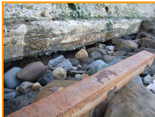
Significant undercutting to defence (Asset Ref. 1221D901D0802C03)
