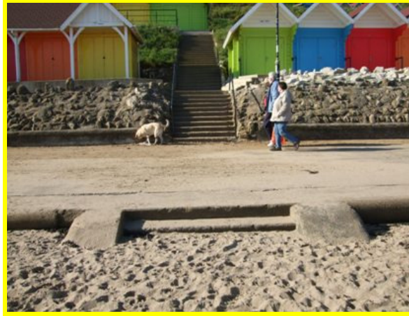
High beach level covering most of stairs (Asset Ref. 1221D901D1201C12001)
