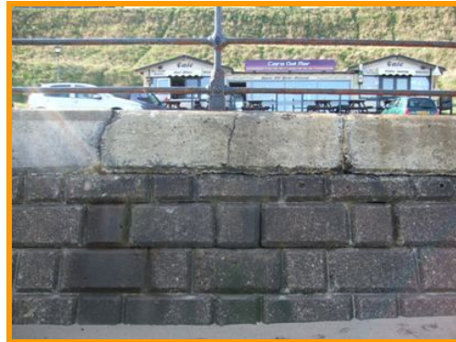
Cracking through and beneath capping, near southern end of defence (Asset Ref. 1221D901D1201C07)
