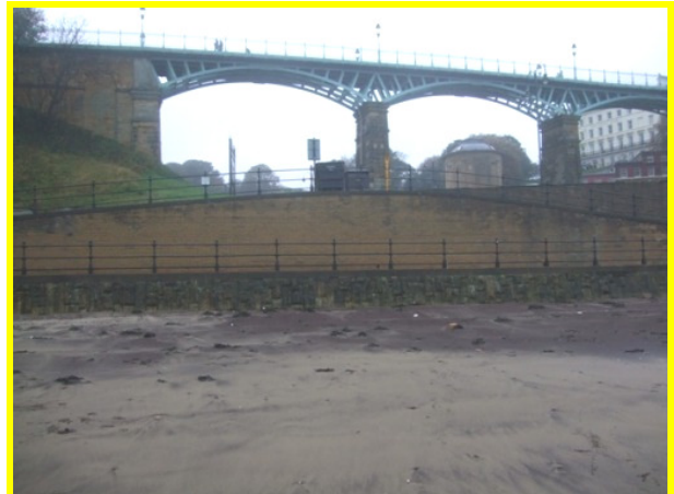
Second stage wall, sea wall and promenade at end of Foreshore Road (Asset Ref. 1221D901D1301C09)
