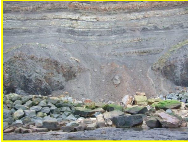
Close up of the base of a rockfall over rock armour defences (Asset Ref. 1221D901D0803C05)
