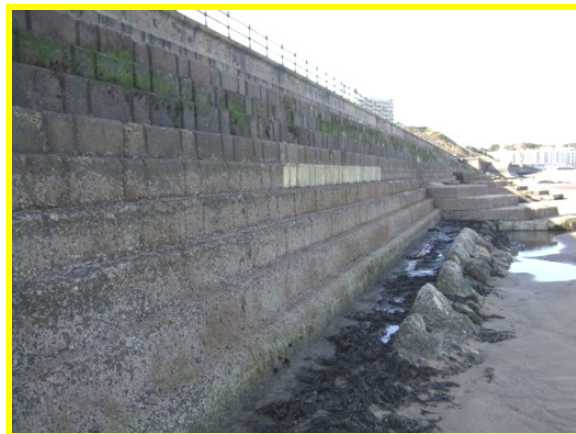
Looking north, showing eroded toe and repairs to blockwork face (Asset Ref. 1221D901D1201C08)
