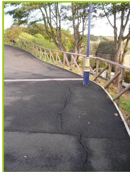
MU28/Y Cracking of footpath (Inactive)
