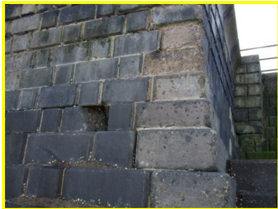
Missing blockwork and damage (Asset Ref. 1221D901D1202C23)
