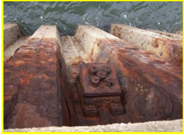
Significant corrosion of steel piling (Asset Ref. 1221D901D1301C17)
