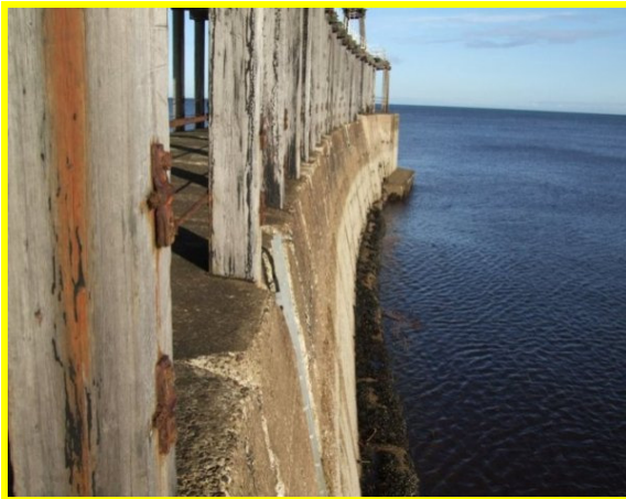
Erosion to edges of west concrete breakwater (Asset Ref. 1221D901D0803C01)
