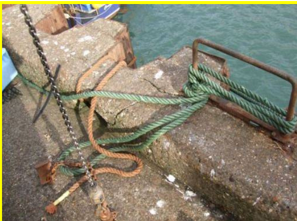
Cracking to concrete capping of sheet piling (Asset Ref. 1221D901D1301C13)
