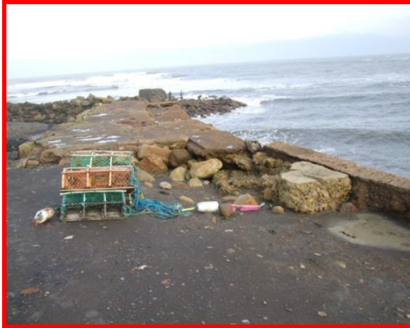
Looking at the end of the breakwater with evidence of erosion and failure (Asset Ref. 1221D901D0502C01)
