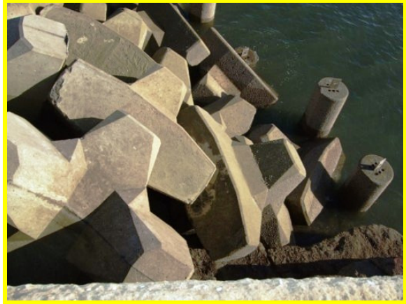
Far end of harbour arm showing potential lack of armour fill (Asset Ref. 1221D901D1301C01)
