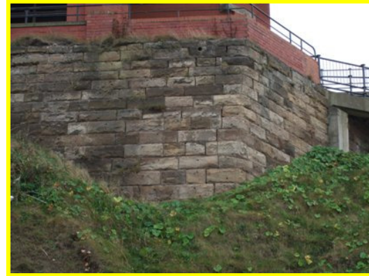
Mortar loss and surface erosion to wall (Asset Ref. 1221D901D0802C15)
