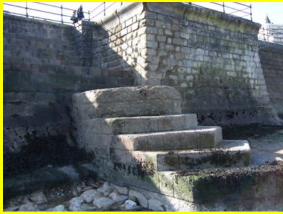
Cracking outbuilt section at north of defence. (Asset Ref. 1221D901D1201C08)
