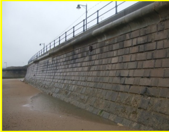
Erosion to sea wall and replaced capping beam (Asset Ref. 1221D901D1602C03)
