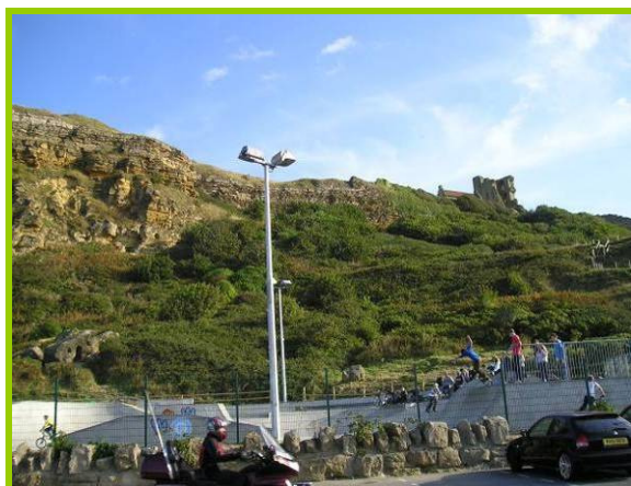
MU21/1 Well jointed hard rock behind the skate park (location of former rockfall) (Inactive)
