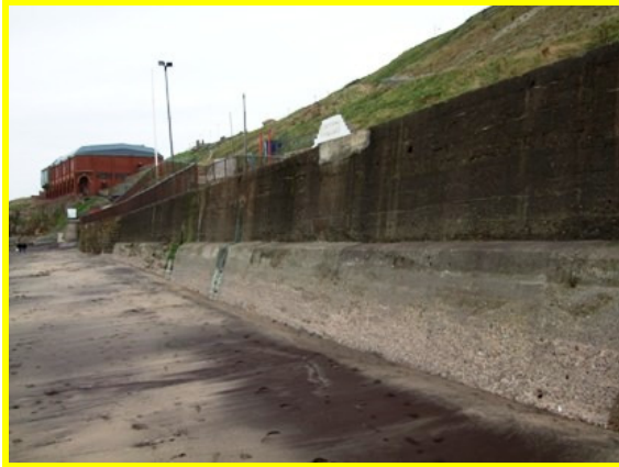
Overview of asset, looking south. Patchwork repairs to capping visible. (Asset Ref. 1221D901D0802C04)
