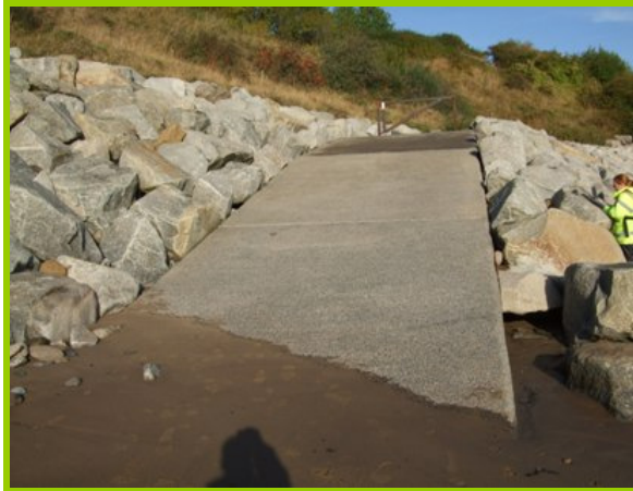
Slipway next to rock armour at south end of bay (Asset Ref. 1221D901D1003C07001)
