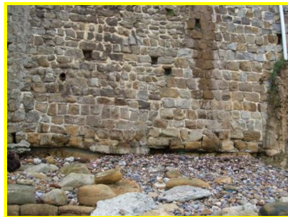
Undercutting to blockwork section, requires repair (Asset Refs. 1221D901D0802C09)
