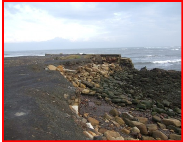
Outflanking and erosion occurring behind the breakwater (Asset Ref. 1221D901D0502C01)
