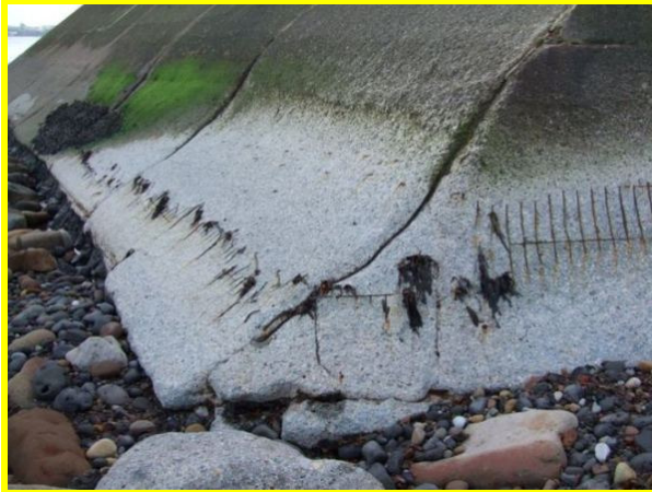
Exposed reinforcement bar and undercutting to concrete revetment (Asset Ref No.1221D901D0701C02)
