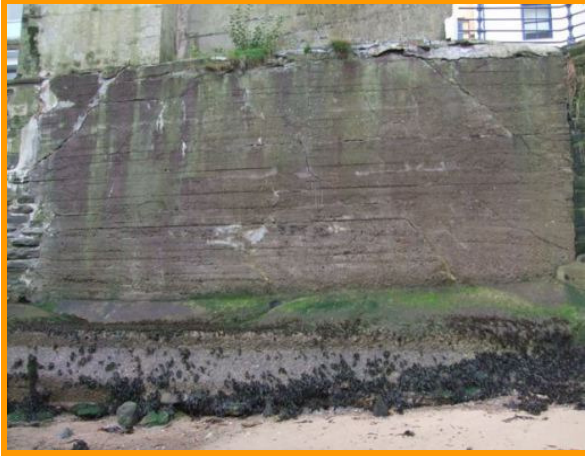
Cracks throughout wall and toe (Asset Ref. 1221D901D0402C22)
