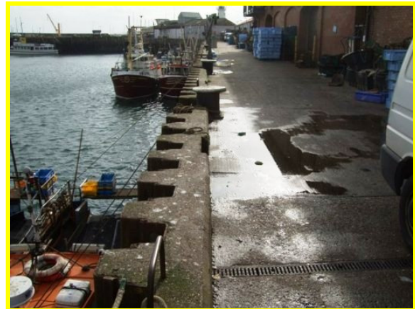
Overview of asset near the market on West Pier (Asset Ref. 1221D901D1301C13)
