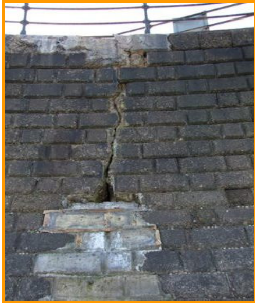
Large vertical cracks running the full height of the sea wall with repair work (Asset Ref. 1221D901D1201C21)
