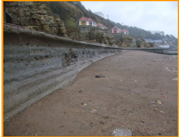
Repaired wall eroded with sections of replaced wall and capping beams (Asset Ref. 1221D901D1302C02)
