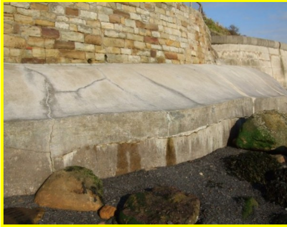
Repaired vertical cracks to toe of wall, and recent horizontal cracks visible (Asset Ref. 1221D901D0601C06)
