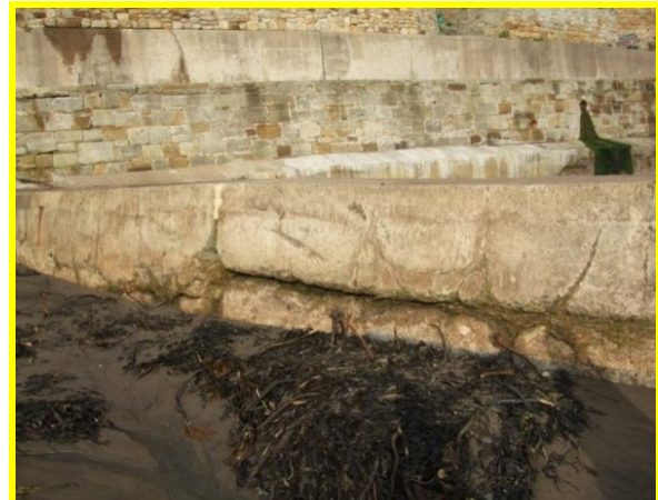
Large horizontal crack to breakwater (Asset Ref. 1221D901D0601C02)
