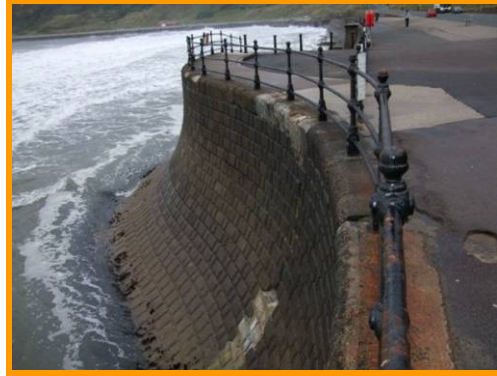
Erosion at joints and repairs to promenade, and damaged coping (Asset Ref. 1221D901D1201C21)
