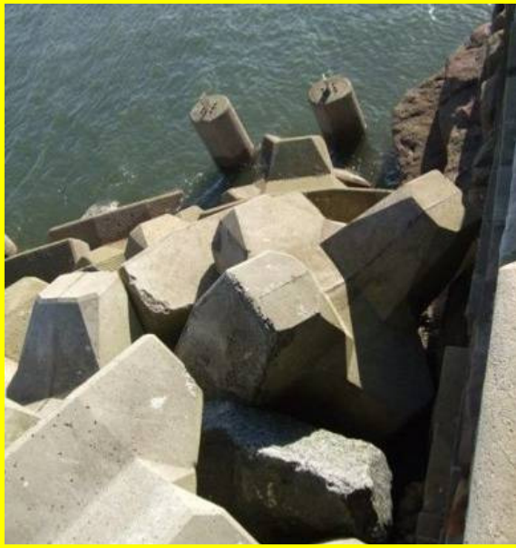
Far end of harbour arm showing potential lack of armour fill (Asset Ref. 1221D901D1301C01)
