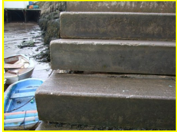
Washout behind steps (Asset Ref. 1221D901D1301C16)
