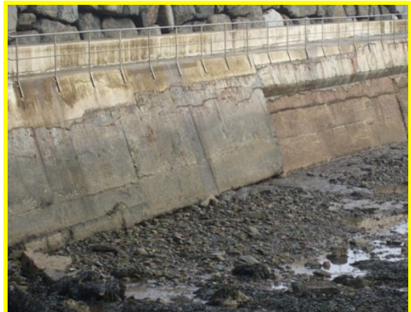
Undercutting occurring to inland part of wall (Asset Ref. 1221D901D0402C01)
