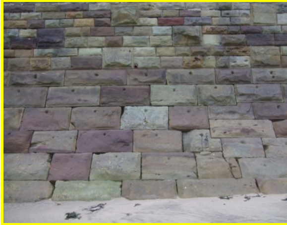
Missing joints throughout blockwork wall (Asset Ref. 1221D901D1301C10)
