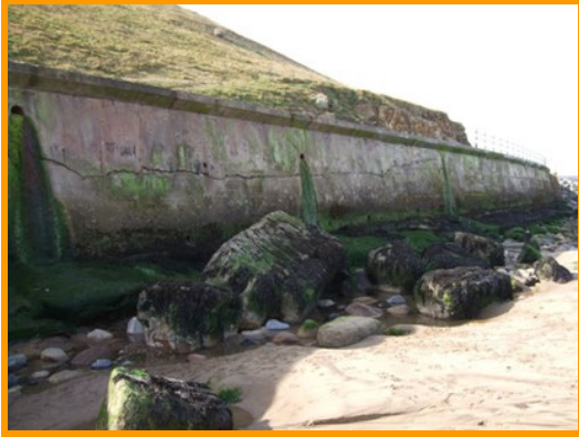
Cracking, repair work and exposed toe (Asset Ref. 1221D901D0802C03)
