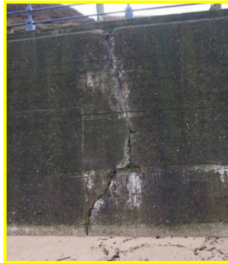
Vertical crack through wall (Asset Ref. 1221D901D0403C01)
