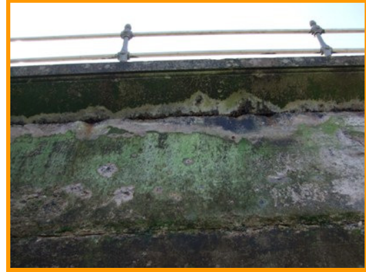
Exposure of rebar and cracking to underside of capping (Asset Ref. 1221D901D0802C03)
