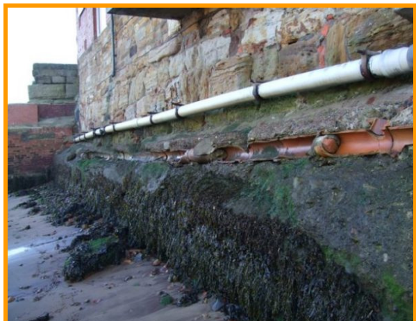
Cracking and erosion to east harbour wall next to breakwater (Asset Ref. 1221D901D0803C08)
