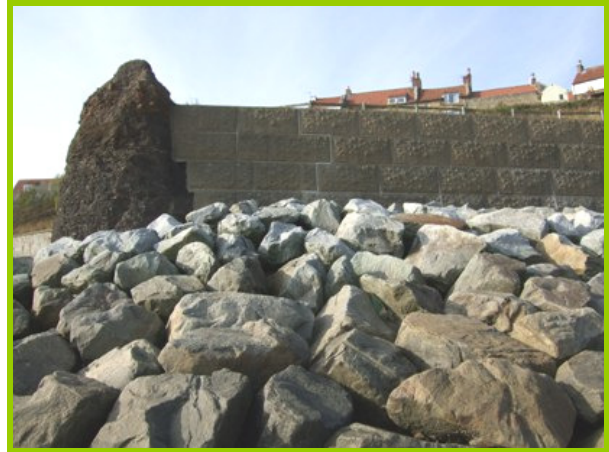
Joint between defended and undefended section. Packing of joints between blocks also visible (Asset Ref. 1221D901D1003C01)
