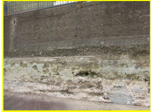
Close up view of eroded front face and significant vertical crack (to left of image) (Asset Ref. 1221D901D0802C04)
