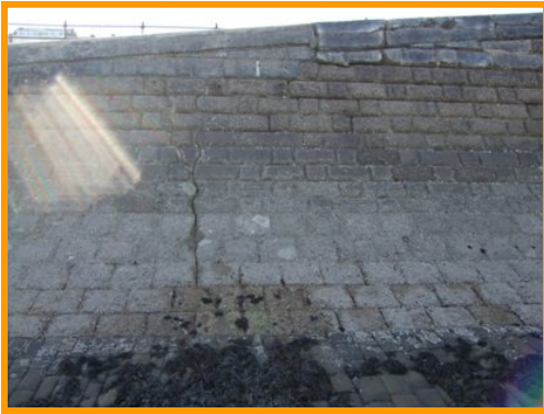
Vertical crack running the full height of the slipway sea wall (Asset Ref. 1221D901D1201C21)
