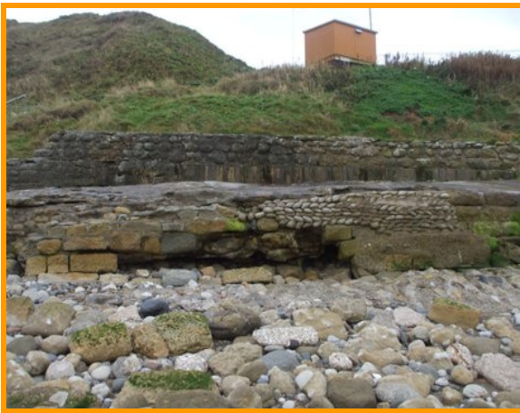
Large voids to makeshift defences to the south of the pumping station (Asset Ref. 1221D901D1402C04)
