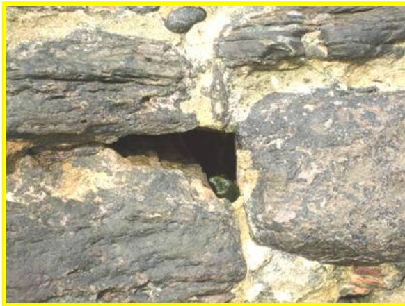
Close up of void (Asset Ref. 1221D901D1003C04)
