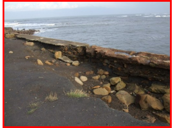
Visible failure (Asset Ref. 1221D901D0502C01)
