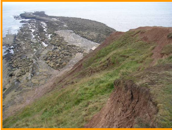
MU27/B Cracking and slumping activity (Partly Active)
