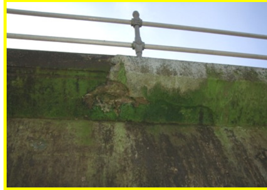
Damage and repair to coping (Asset Ref. 1221D901D0802C01)
