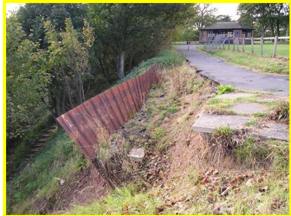
MU28/Z Ongoing slope instability and footpath closure (Locally Active)
