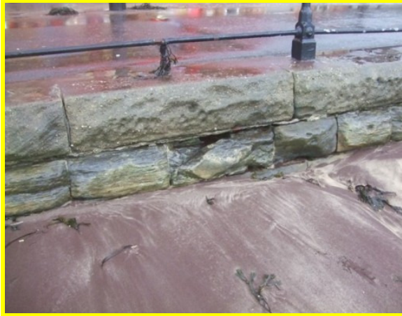
Missing joints and erosion to top part of wall (Asset Ref. 1221D901D1301C15)
