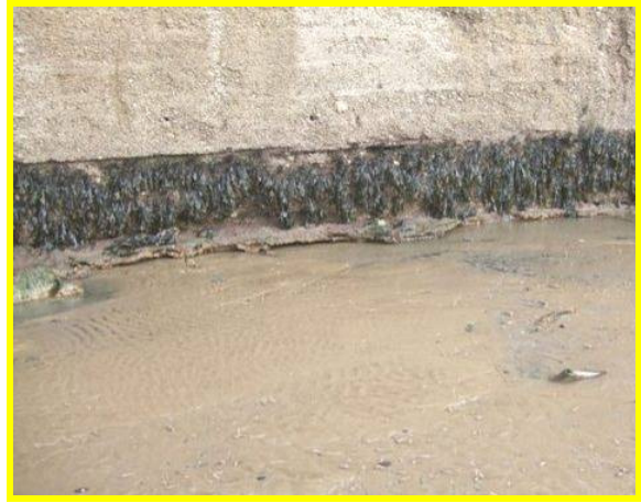
Exposed toe (Asset Ref. 1221D901D1301C07)
