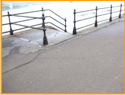
Erosion at joints and cracking to promenade (Asset Ref. 1221D901D1201C07)
