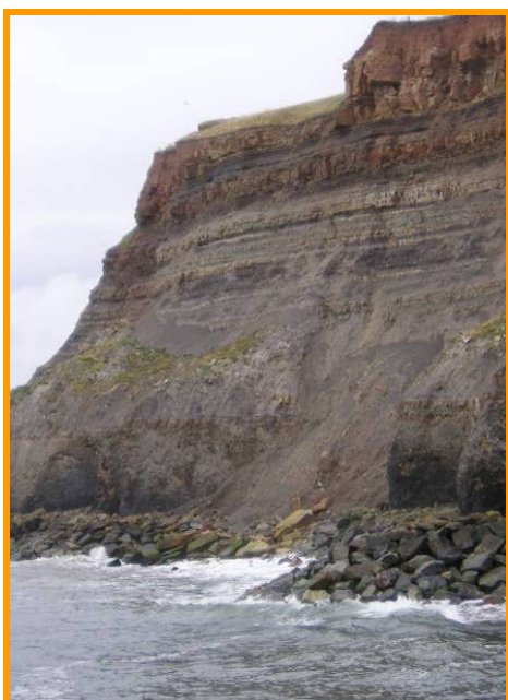
MU12/2 Recent rockfall evidence (Partly Active)
