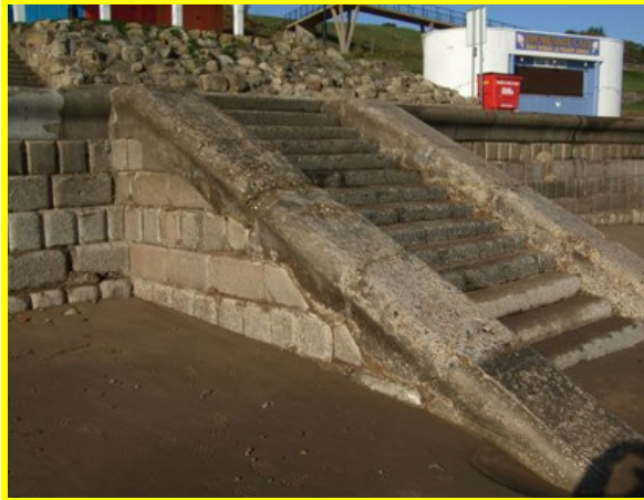
Erosion evident to stairs and side walls (Asset Ref. 1221D901D1201C26001)
