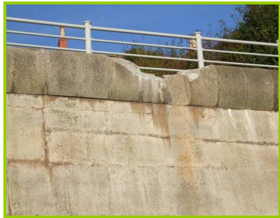
Sea wall with damaged capping beam (Asset Ref. 1221D901D1003C10)
