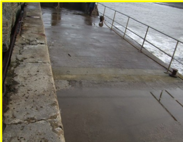
Cracking to beam next to rock armour (Asset Ref. 1221D901D0402C01)
