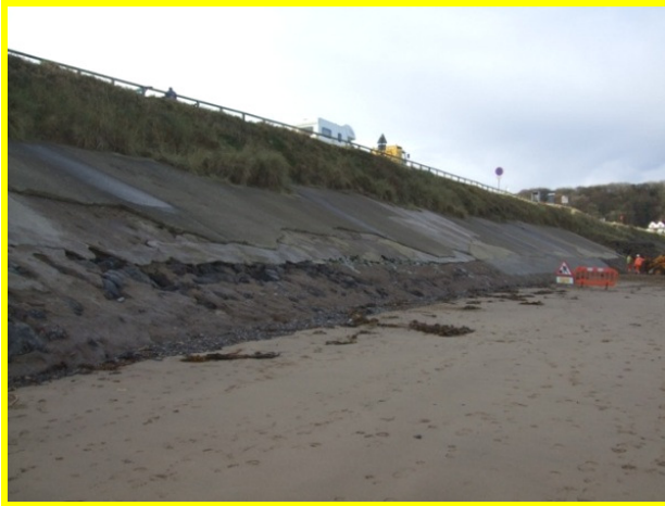
Exposed rock armour at base of concrete revetment (Asset Ref. 1221D901D0702C02)
