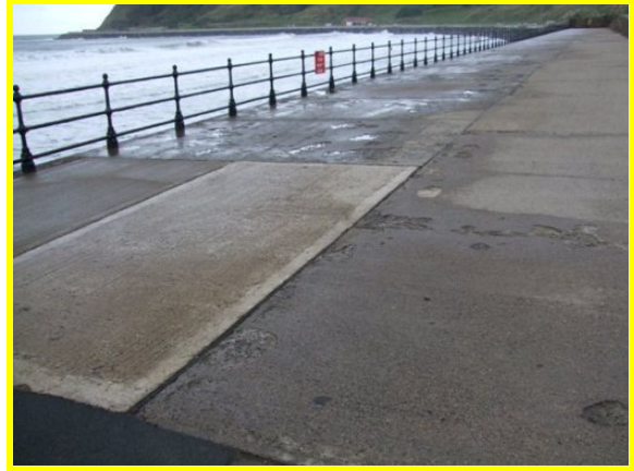
Repaired and damaged promenade, with cracking throughout (Asset Ref. 1221D901D1201C08)
