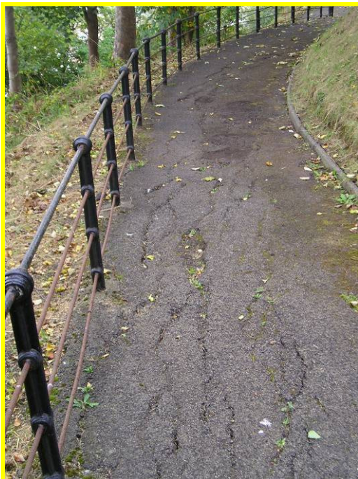
MU22/2 Extensive cracking to footpaths (Locally Active)
