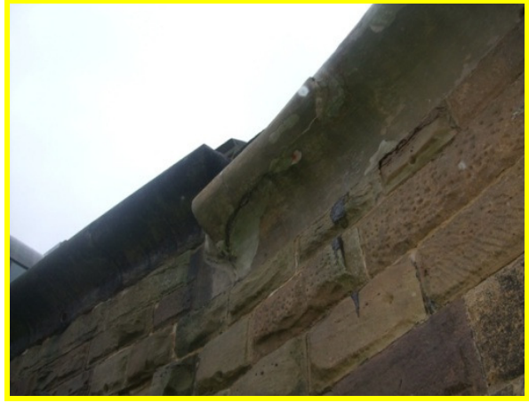
Cracking to the splash beam (Asset Ref. 1221D901D1301C28)
