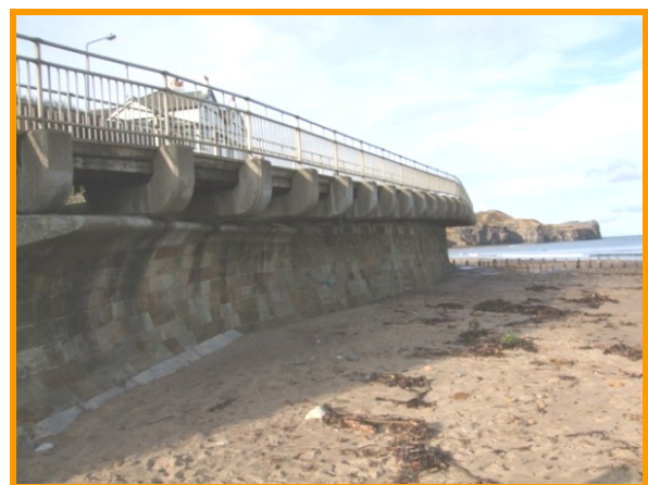
Relatively new blockwork sea wall with undercutting at the toe (Asset Ref. 1221D901D0702C04)
