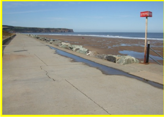
Cracking and settlement of promenade (Asset Ref. 1221D901D0801C01)
