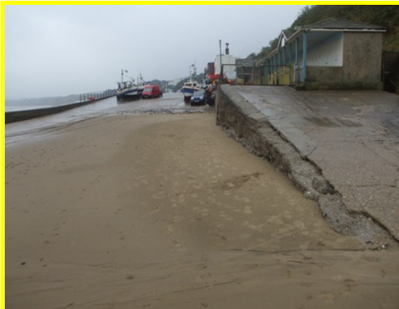
Erosion to the slipway wall (Asset Ref. 1221D901D1602C09002)
