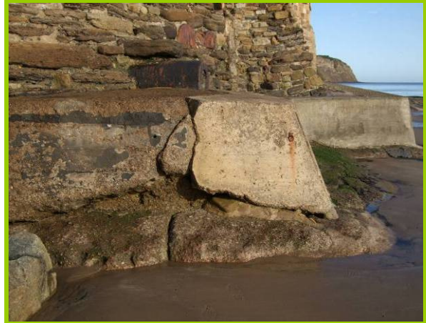
Wide cracks to toe of wall (Asset Ref. 1221D901D1003C06)
