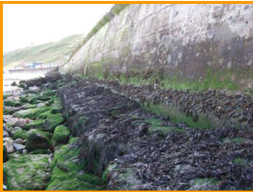
Overview of asset looking south, showing exposure of toe. (Asset Ref. 1221D901D0802C03)
