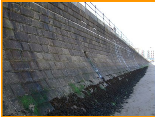
Looking northwards along wall, with filled lateral joints visible (Asset Ref. 1221D901D1201C07)
