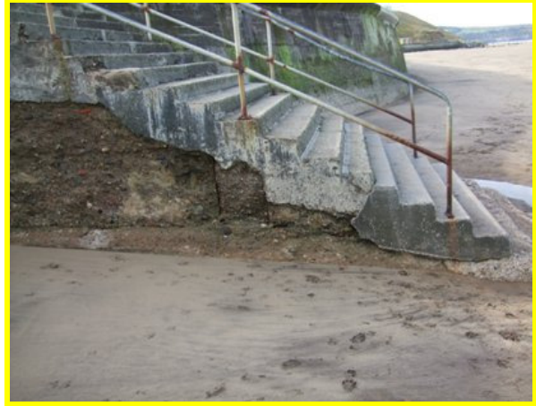
Erosion and cracking to stair side wall (Asset Ref. 1221D901D0802C04001)
