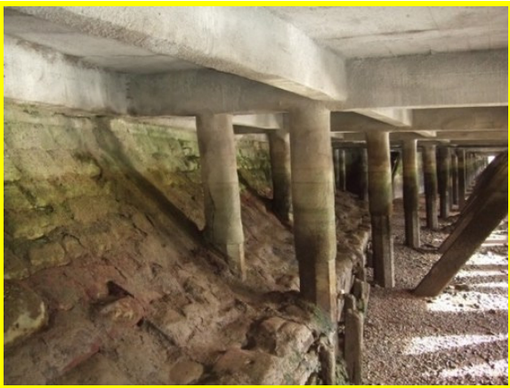
The original quay wall beneath the newer concrete jetty (Asset Ref. 1221D901D1301C06)
