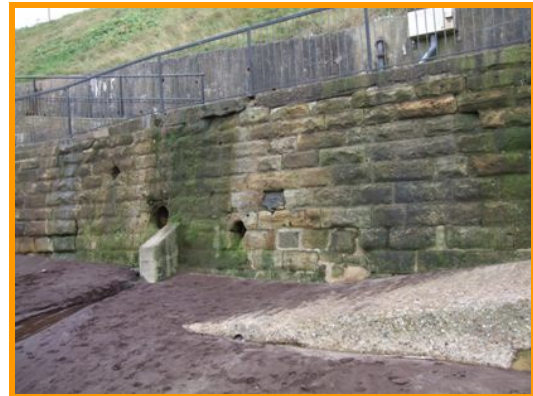
Cracking, mortar loss, damage to capping and localised repairs (Asset Ref. 1221D901D0802C07)
