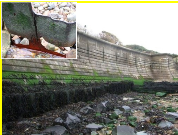
Exposed sheet pile toe (Asset Ref. 1221D901D1201C02)
