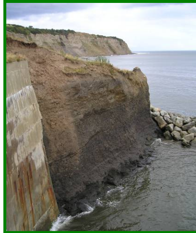
MU16/2 undefended section subject to marine action and potential instability if not addressed (Dormant)
