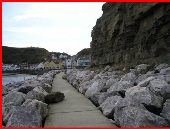
MU4/1a – Rockfall onto the walkway at the eastwards facing end of Cowbar Nab (Totally Active)
