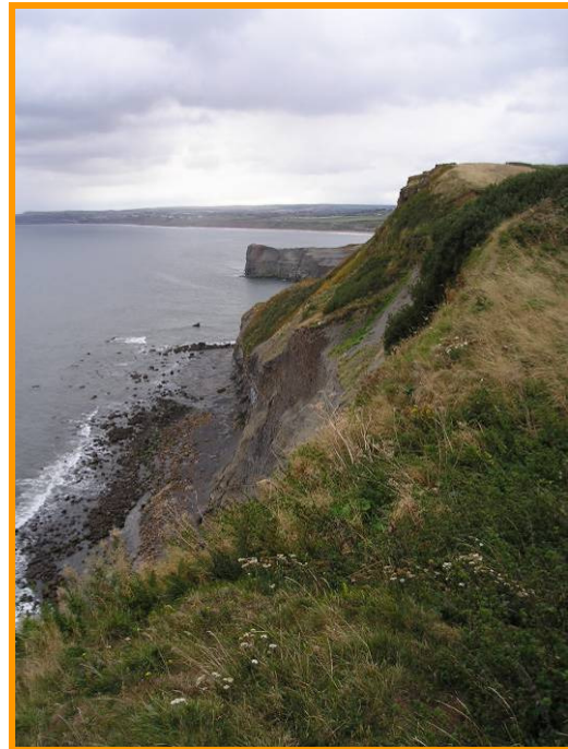
MU8/12 Steep, unvegetated lower slopes and shallower, partly vegetated upper section (Partly Active)
